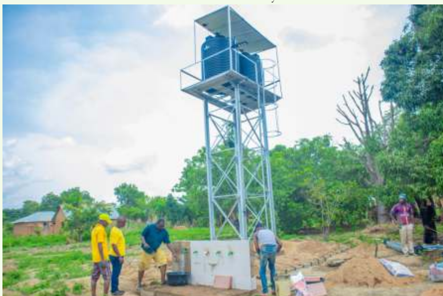
Completed Solar Powered Borehole
